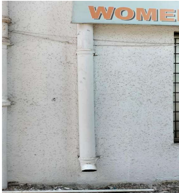
Photo-7: View rain water collection from building for charging the bore
