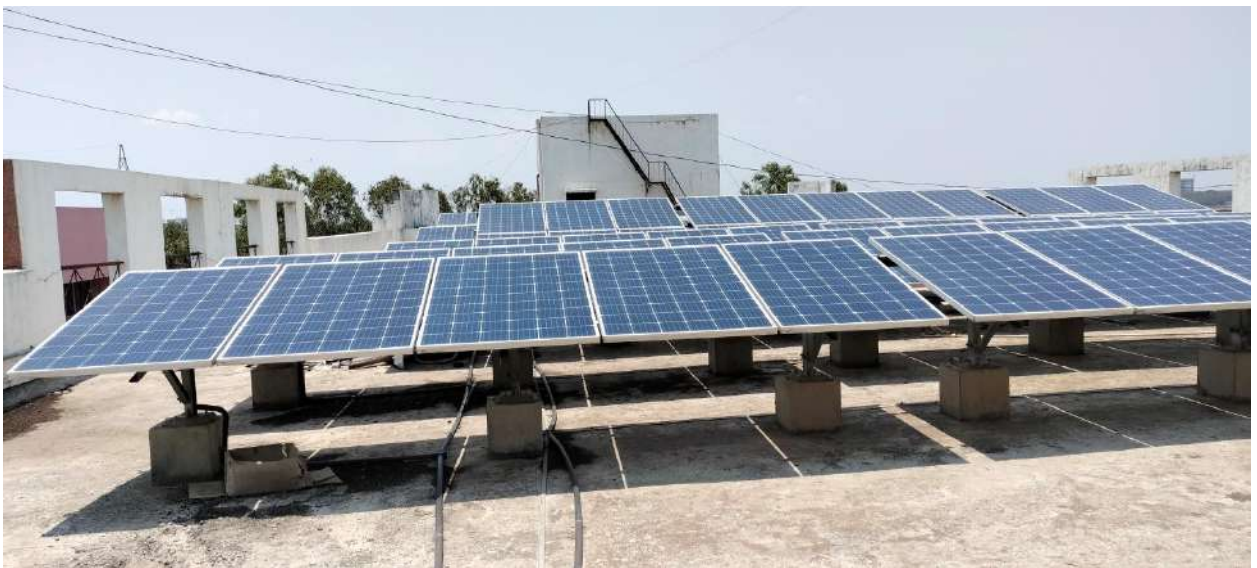
Photo-5: 50 kW solar roof top on hostel building roof.
