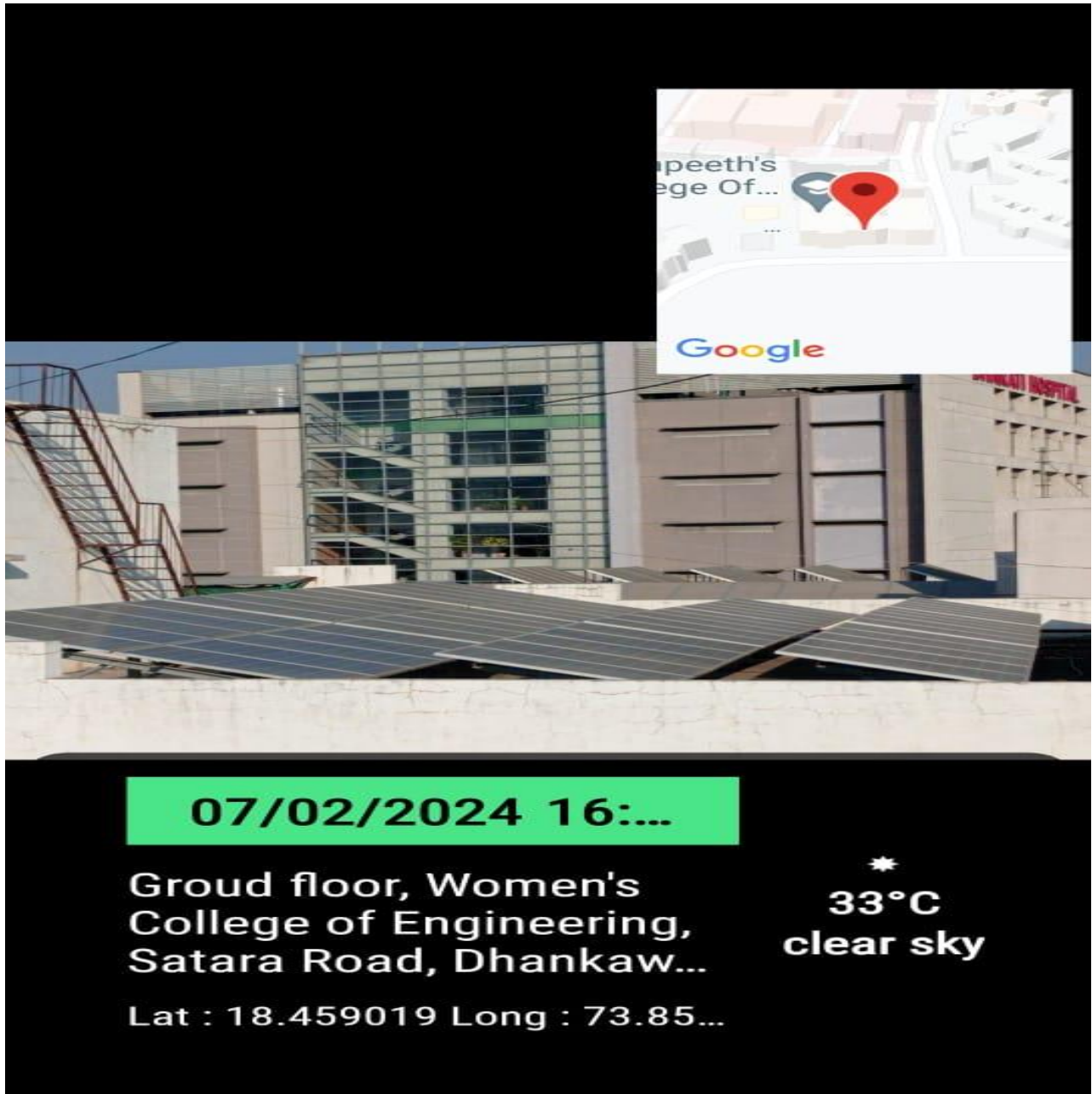
Geotag Photograph for Roof Top Solar Panel View 2
