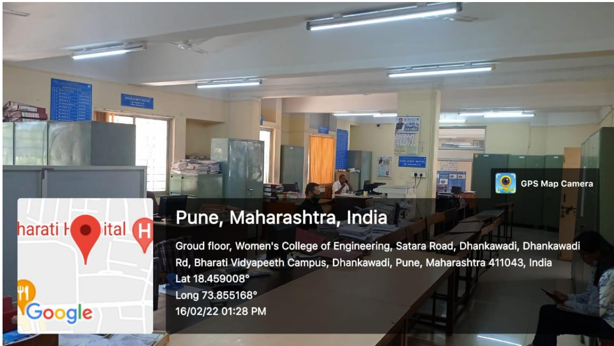
Geo tagged Photograph for use of LED tube lights installed at Administrative office of the institute
