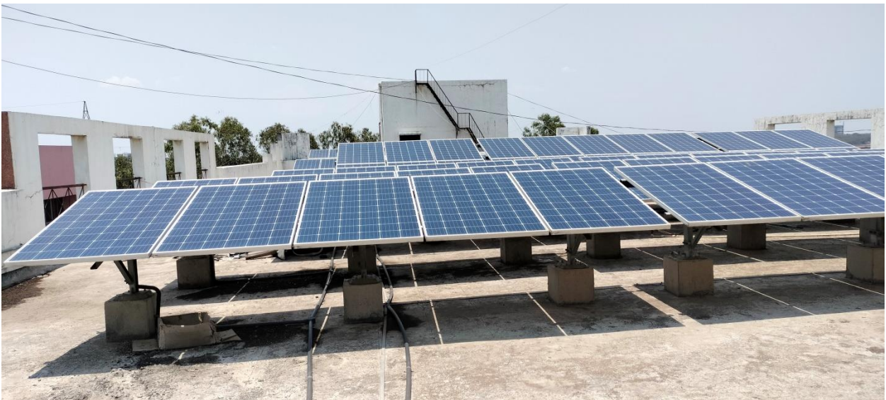
Photo-2: 50 kW solar roof top on hostel building roof.
