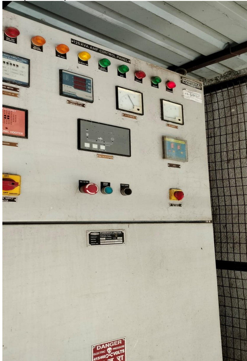
Photo-1: APFC 125kVAR at Bharati Vidyapeeth's College of Engineering campus
